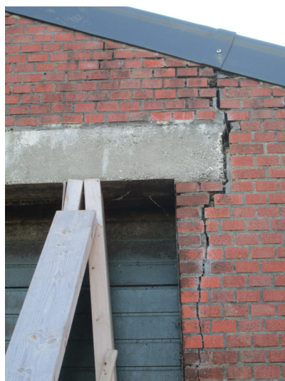
Figure.22: Tear at the lintel of barn entrance in Loppersum | own image
