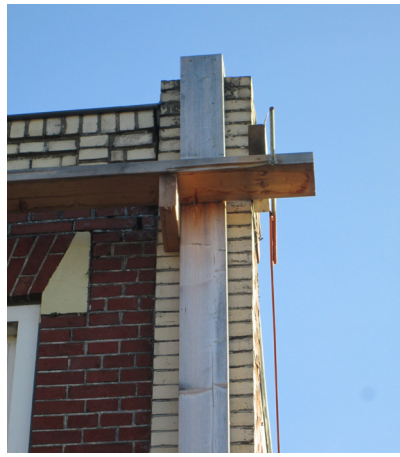
Figure.19: Tensile anchor to prevent the facade from falling over | own image
