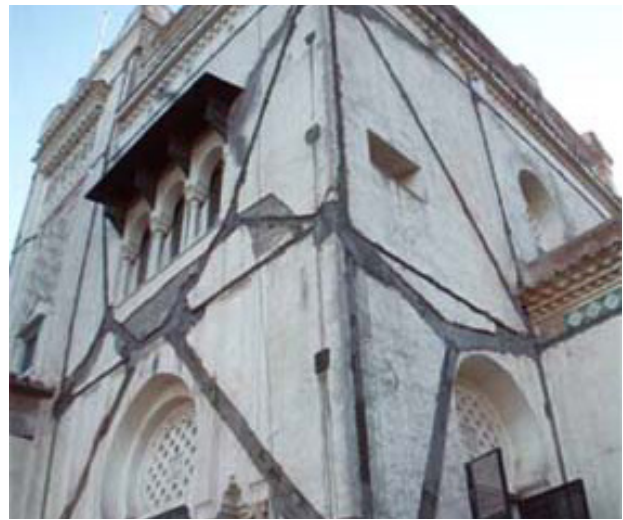
Figure.57: Implementation of dampers into brick wall of an embassy building | Source: : DC 90
