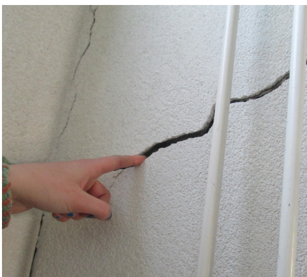
Figure.63: Tear in the interior of a home | own image
