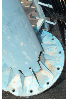
Fig. 2. Detail of the rupture at mid-height
