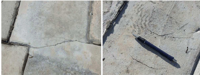
Figure 2-23 Cracks in concrete
