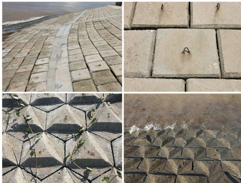
Figure 2-21 Irregular placement of blocks
