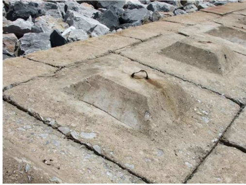
Figure 2-20 Rust of the transport ring
