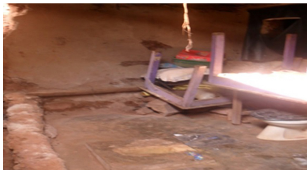
Fig. 4. Full pit latrine in the Biryogo settlement (used as a store of miscellaneous equipment next to a living room).
