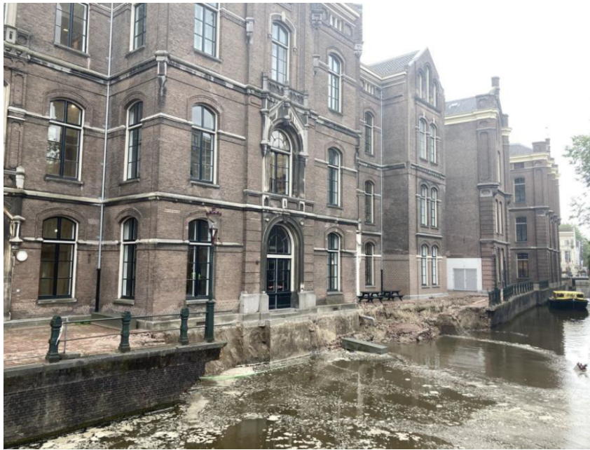
Figure 3.1: Collapse of Grimburgwal in 2020. [25]
