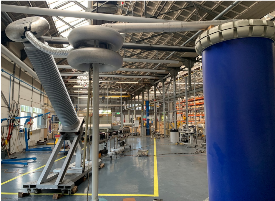
Figure 6.24: Voltage application to the test object
