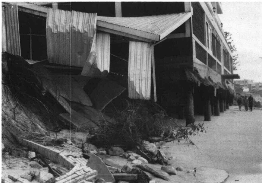
Figure B3.1 Storm Damage to Beaches and Coastal Structures, New South Wales.
