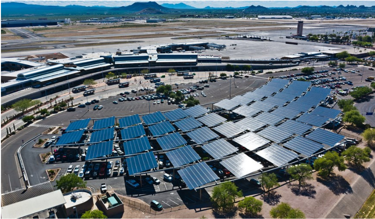
Figure 1.2: PV System at Tucson International Airport, USA [7]
