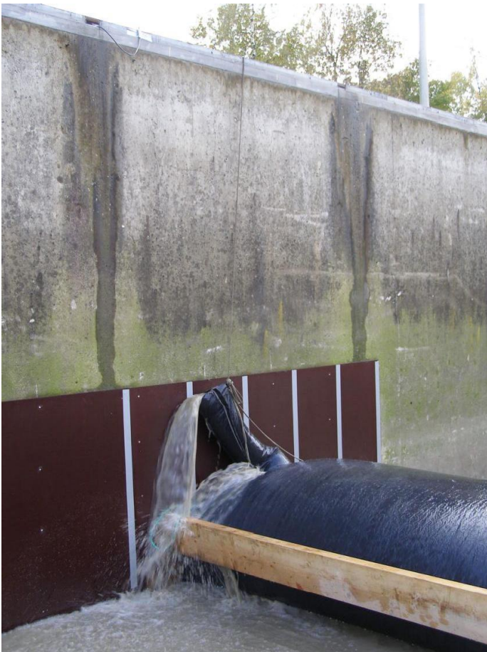
Photo 14: Filling (over pressure) hose
