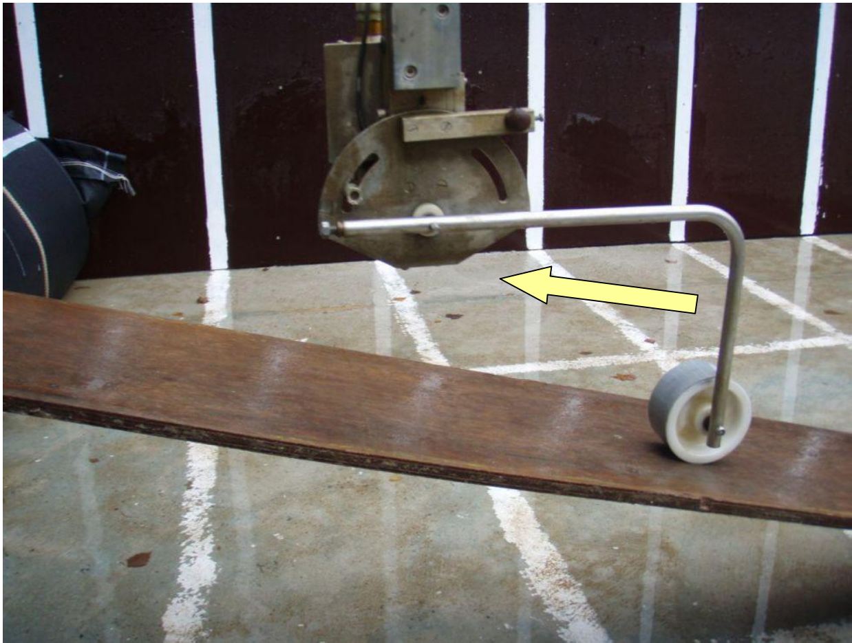
Photo 19: Use of a slat at the landside to prevent damaging the profiler and geotextile tube.
