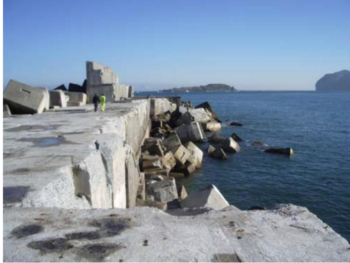
Figure 7. Port of Bermeo, Biscay (northern Spain). Slide failure and overturning in 2010. Source: (Negro Valdecantos et al., 2013).
