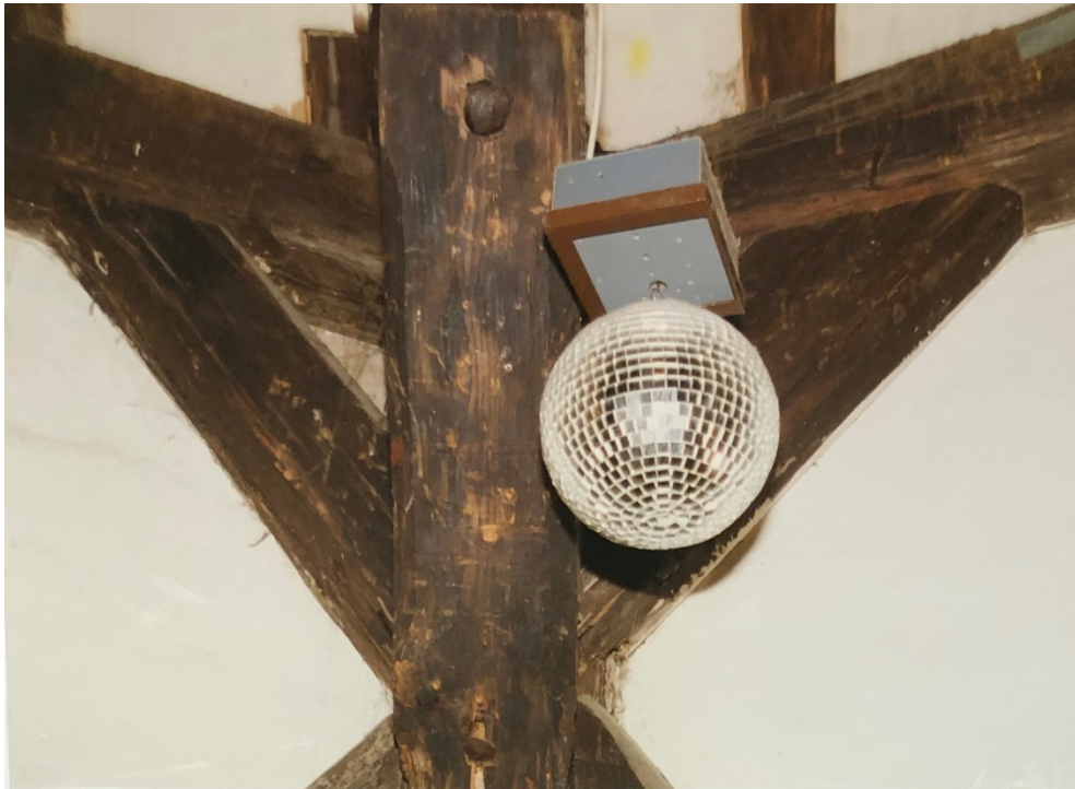
Fig. 1. Photographic documentation of the lantern roof structure in the Dicker Turm, showing diagonal bracing of the posts and the later disco-ball installation. Building Archive Görlitz, Grdb.-Nr. 10690, Bauakte Bd. 1, p. 18.
