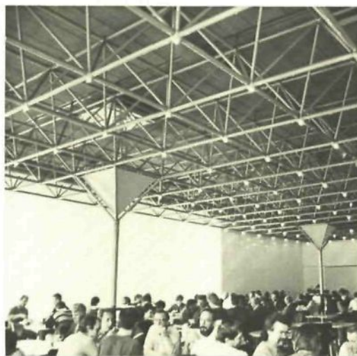
94 Tuball space frame for Auping, Deventer NL. Module 1.2 m, combined with hardly visible halogen lamps in all lower chord nodes. Architect Roeterdink of Postma Partners, with industrial designer Frans de la Haye.
