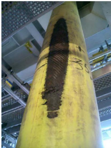
Fig. 5. Damaged outer sheath.
