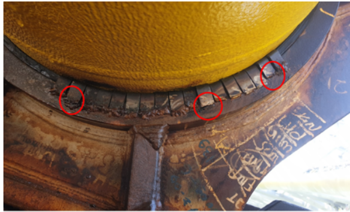
Figure 6.6: Shim plates applied to support structure at saddle
