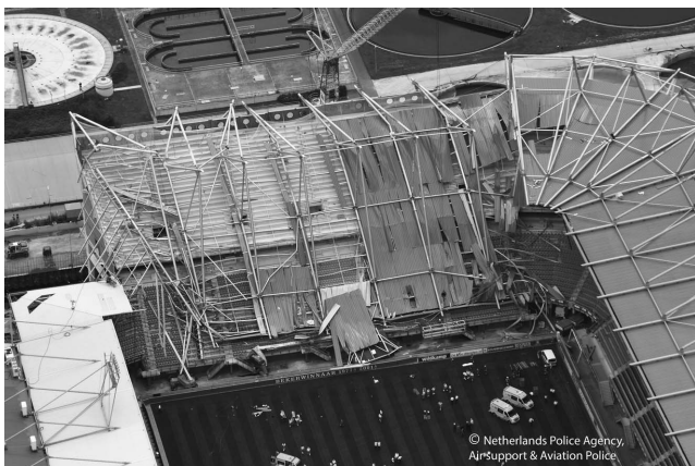
Figure 3. Roof of FC Twente stadium after collapse (reproduced by permission of Netherlands Police Agency: Air Support and Aviation Police)
