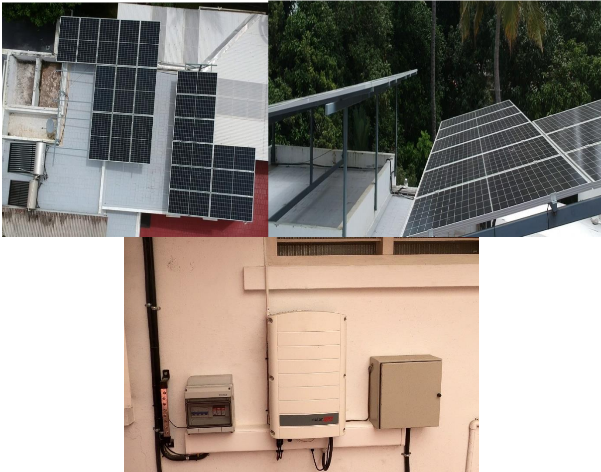
Figure 7: Typical rooftop Solar PV installations and BOS in India (Photo by Author taken in Kerala, India (25 July 2020))
