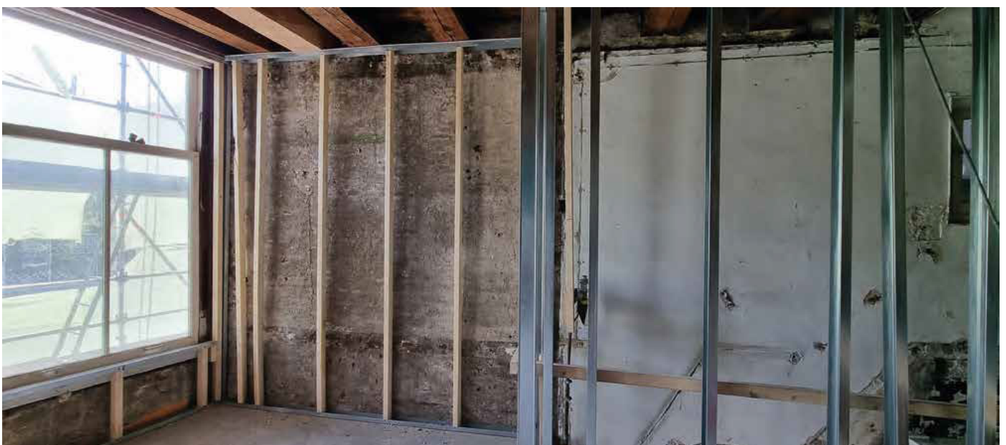
Figure 25: Standard insulation layer applied to the interior in the form of insulated cladding (Veldt, 2022)
