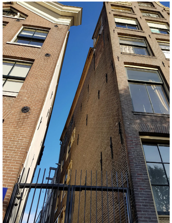
Figure 21: Inclination of the building (Buro Van Stigt, 2024)
