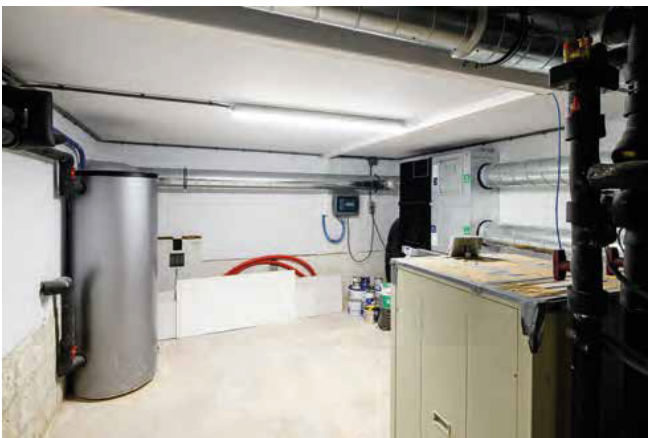
Figure 30: HRV ventilation system on the right side of the basement (Veldt, 2022)
