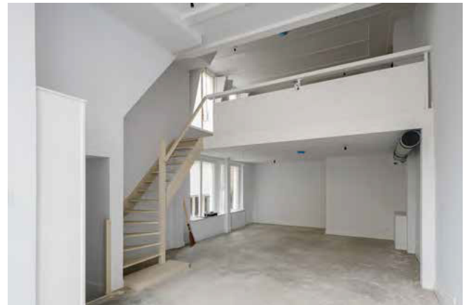
Figure 7: Additional floor was inserted, known as a “hangkamer” or “insteek” (Oudezijds Voorburgwal 136) (Veldt, 2022)
