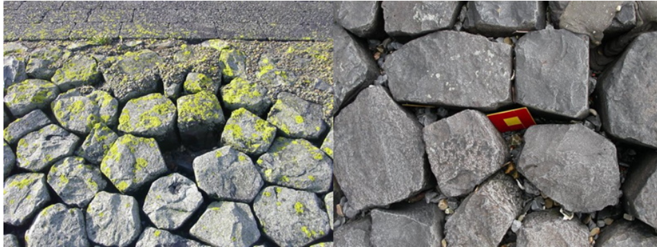
Figure 1.1: Damaged pattern-placed revetments, left: a missing element, right: washed-out joint filling (Waterschapshuis, 2019)
