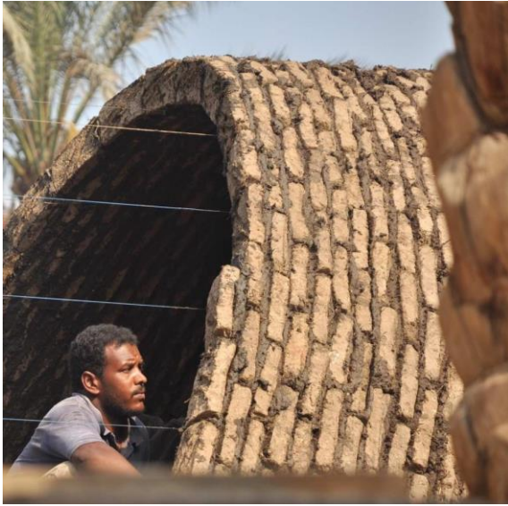
Nubian vault under construction showing guide lines for form, Aga Khan Award for Architecture (2009)
