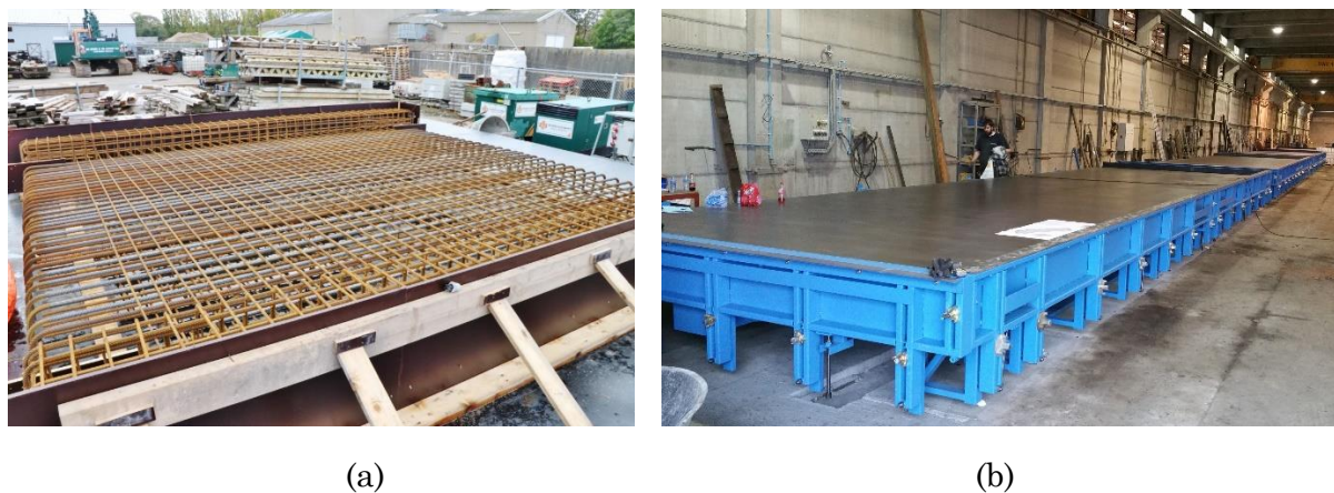
Figure 2.2 : Two main types of formworks used for solid slab bridge designs: (a) timber formwork used for in-situ casting; (b) steel formwork used for prefabrication (photo credit: (a) De Boer & De Groot; (b) Cometal).
