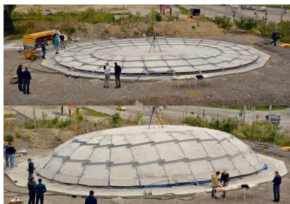
Figure 2.12 : Experiment on pneumatic forming of hardened concrete at the Vienna University of Technology (Kromoser & Kollegger, 2014)
