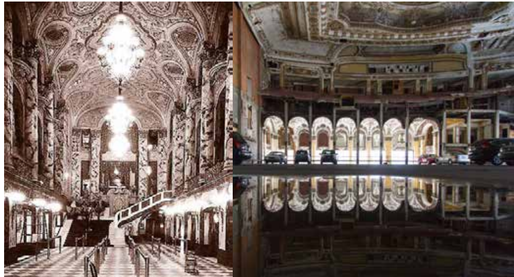
2-3. The world's finest Renaissance parking garage: the former Michigan Theater from the glorious days of Detroit. After a series of unsuccessful transformations the building was badly damaged and left to fall into decay. Now the remnants of the theater serve as a covered parking lot (Rogers, 2010). Source: Rogers (2010) and Vanessa (2012).
