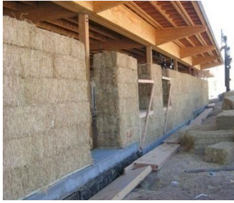
Figure 2.9, application of straw bales in the Santa Clarita Transit Maintenance Facility designed by HOK , source: .inhabitat.com/2007/10/25/hoks-lead-gold-certified-straw-bale-building
