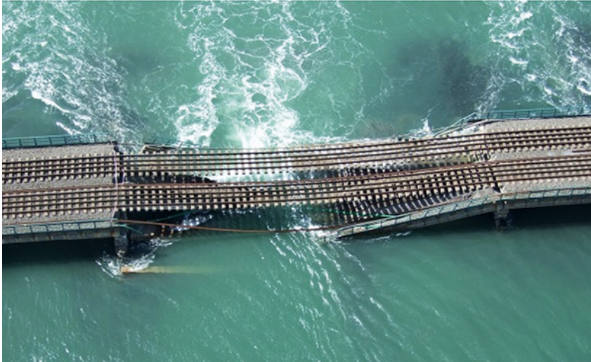
Figure 1. Malahide Bridge Collapse (21 st of August 2009)
