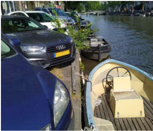
(a) Quay wall horizontal movement and tilt, a tilt between 4-5 degrees has been observed.
