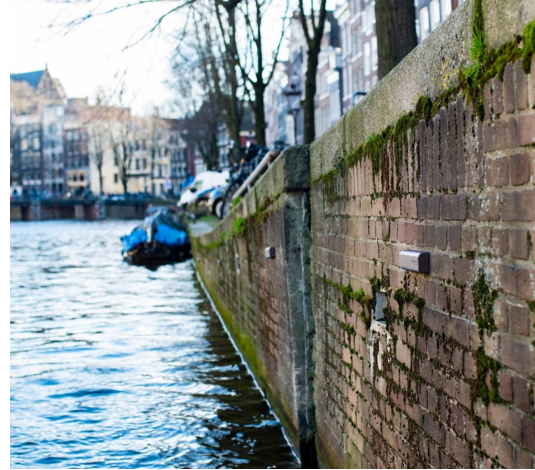
(b) Forward tilt of the quay wall at the Singel, Althen Sensors
