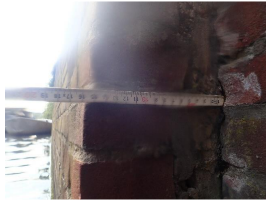
(b) Quay wall horizontal displacement, around 15 cm.
