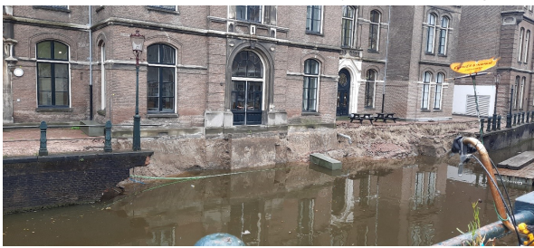
(c) Collapsed quay wall at Grimburgwal, (Korff et al., 2022)
