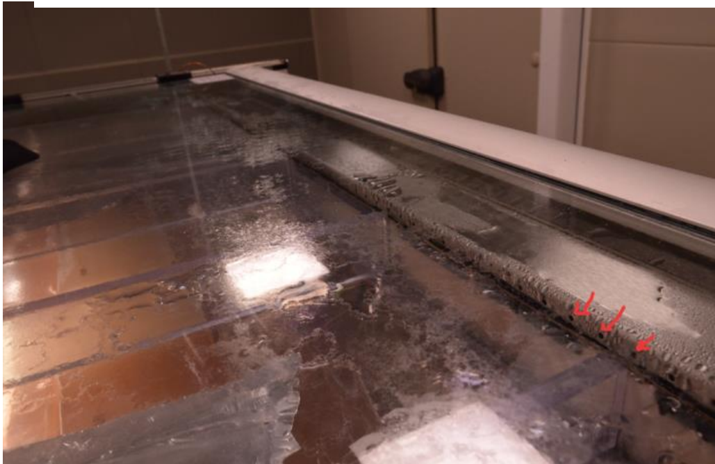
Fig. A3. Circular perforations (as indicated by the red arrows) that were added to the upper fan room to mitigate the condensate film.
