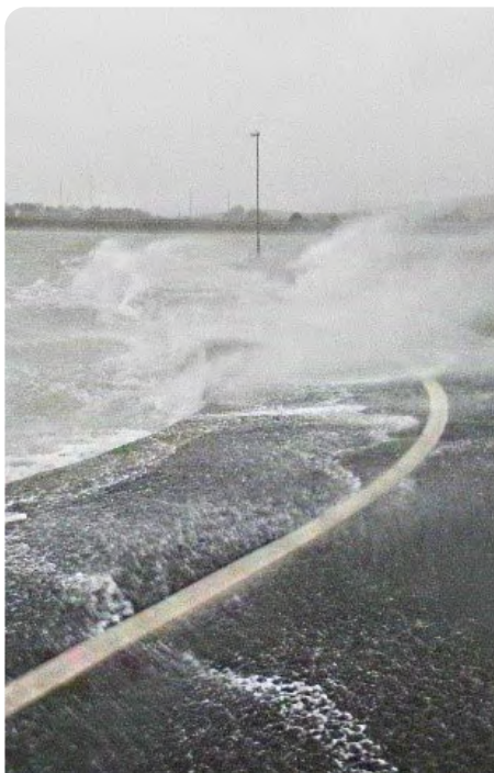
Wave overtopping on a grass-covered dike with a road on top. Photo via https://coastalpartners.org.uk/ .
