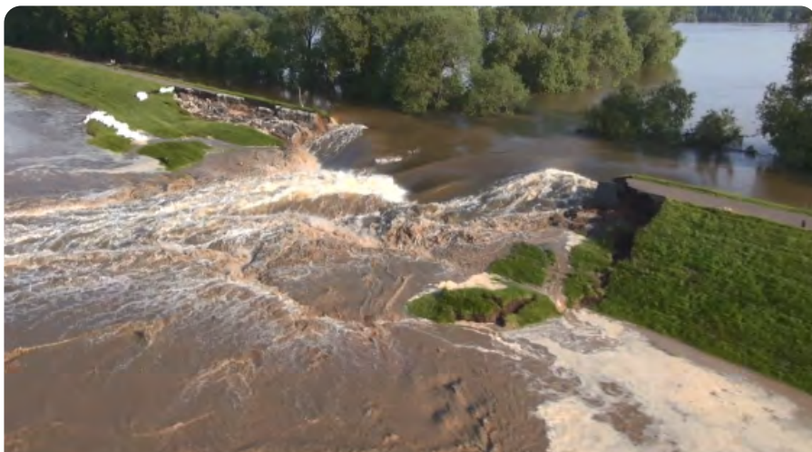
Dike breach caused by inner slope instability. Photo by Weichel (2013).
