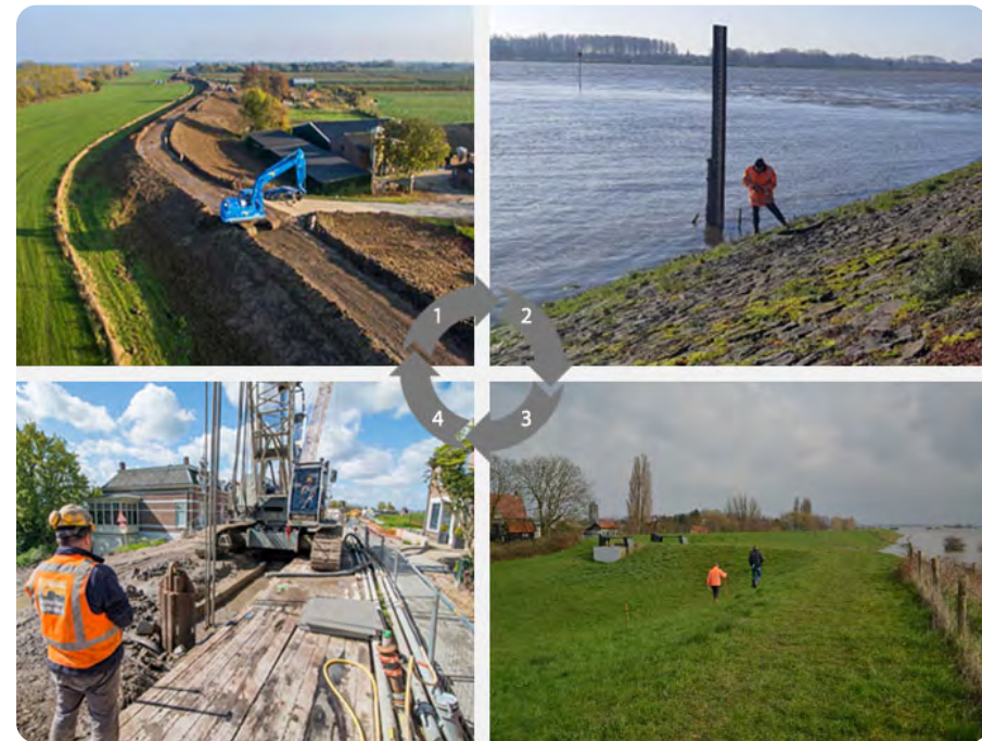
Figure 2: Example of the activities to ensure life-cycle performance: photo 1 and 4 reinforcement, 2 and 3 inspection. Photos by HWBP (2018, p.103) / Pascal Ogink, Wouter Jan Klerk, Mark van der Krogt and the Flood Protection Programme, respectively.
