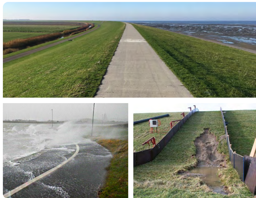
Figure 2: Top: Road on a grass-covered sea dike. Photo by Vera van Bergeijk. Bottom-left: Wave overtopping on a grass-covered dike with a road on top. Source: https://coastalpartners.org.uk/ . Bottom-right: Erosion of the grass cover at the inner toe during field tests. Source: Hoffmans (2014).
