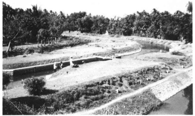
Figure 2 Vortex tube installed in canal in Java showing waste channel discharging into settling basin
