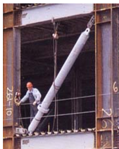
Figure 3.31: A Diagonal Viscous Damper installed in a building
