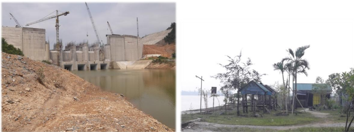
Figure 4: Construction of reservoirs (left) and recently flooded houses (right).
