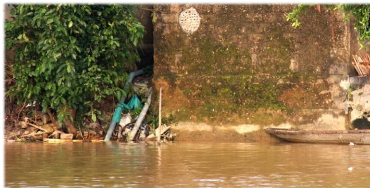
'Hidden' sewage pipes in the river.
