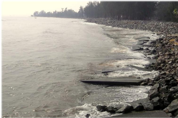
Broken revetments near the west jetty of the Thuan An inlet.
