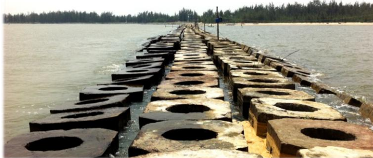
The west jetty, build with a modified Haros, looking towards the shore.
