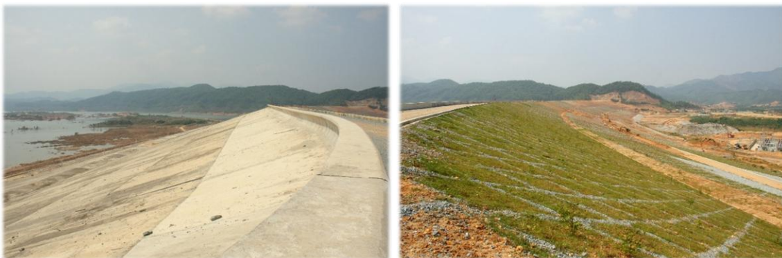
Figure 24: Ta track main dam, upstream side (left) and the downstream side (right).
