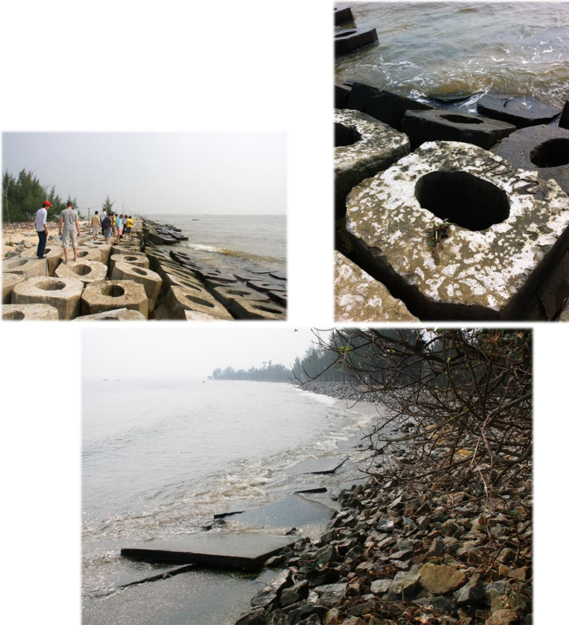
Figure 8: Modified Haros' placed without foundation (upper photos). The west jetty as a whole looks like a bunch of randomly placed armour units. Near the west jetty broken revetments can be observed (lower picture).
