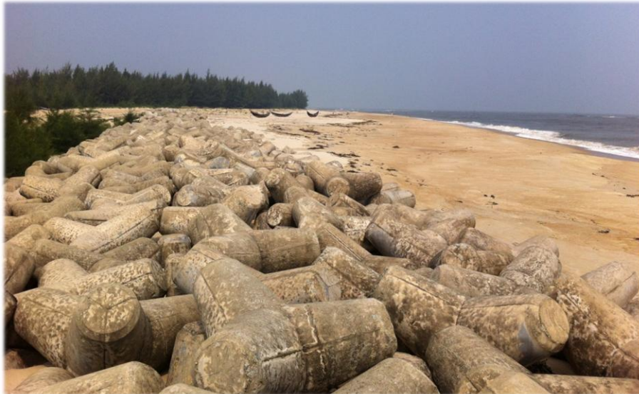
Figure 9: Tetrapod breakwater, with Tetrapods of 1.5-2.0 metres high placed quite regularly.
