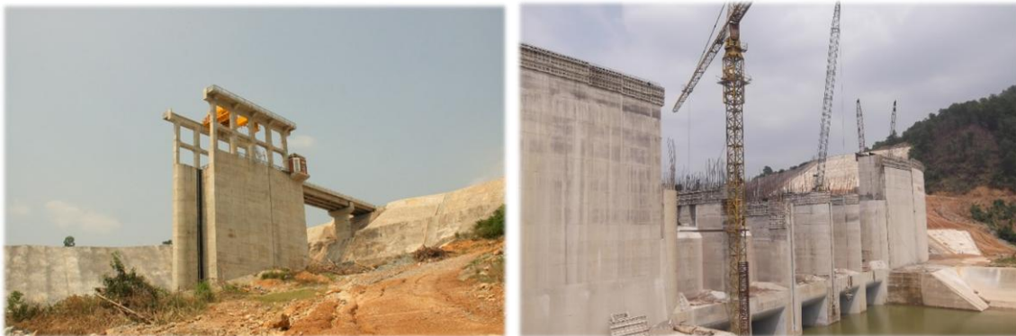
Figure 25: Ta Trach hydropower construction (left) and Ta Track spillway under construction (right).
