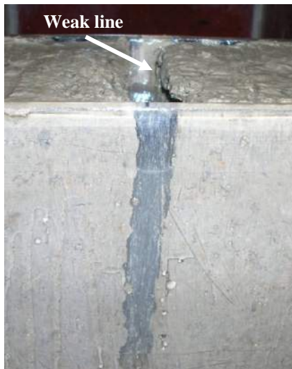
Figure 4-1 Water filled crack with its weak line as the result of imperfect cracking process.
