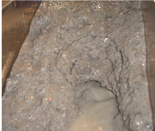
Figure 4-15 Sand undermining causes more damages to the clay cover
