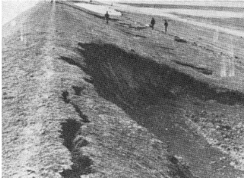
Figure 2-7 Damage at the sea side of a dike due to breaking wave impacts (Stephan, 1981)
