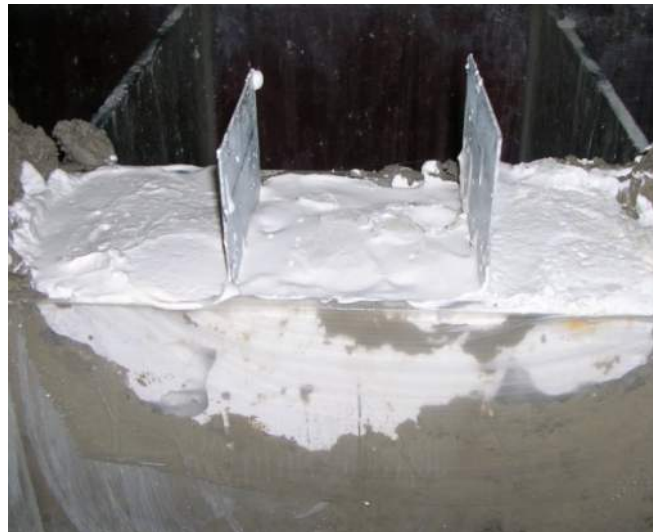
Pouring the gypsum into the scour hole and dividing it into 3 sections by partitions
