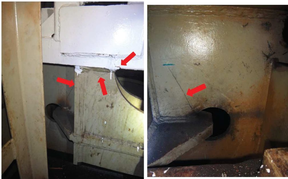
(a) Picture of the cracks in the gearbox foundation of the cutter ladder. (b) Picture of the cracks in the thrust bearing foundation.
