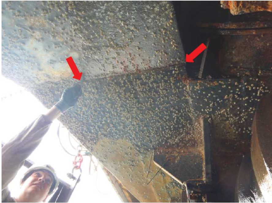
Figure D.1: Picture of the damage to the bottom of cutter ladder, employee for scale
