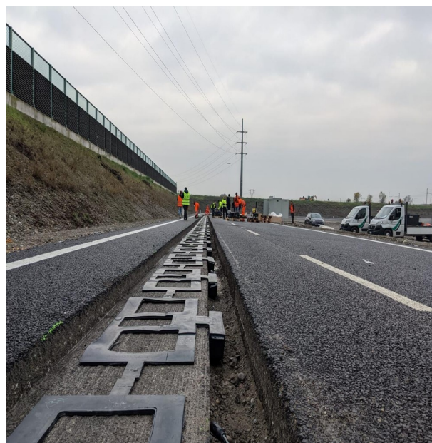
Figure 5.5: Inductive coil of in-road inductive technology (photo from Electreon)
