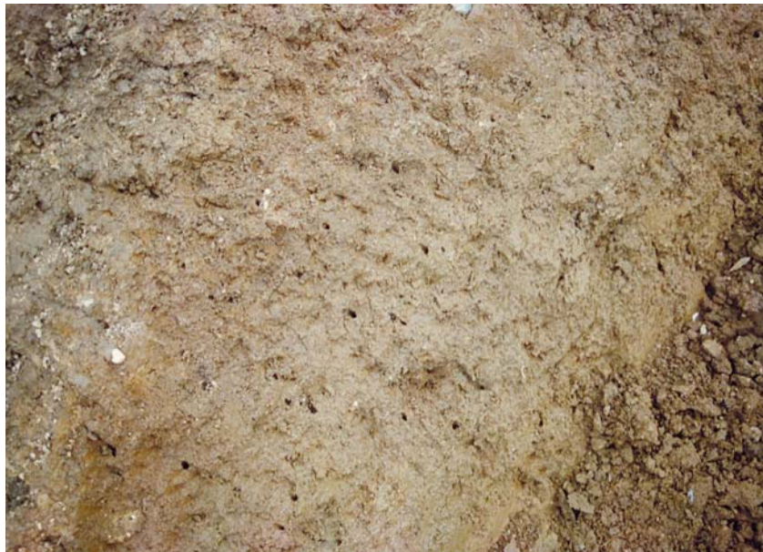
Figure 3.6: Worm tunnels in a dike core at Hank, 2 m below the crown: the worm tunnels were found in large numbers up to 0.6 m above the local groundwater level.
