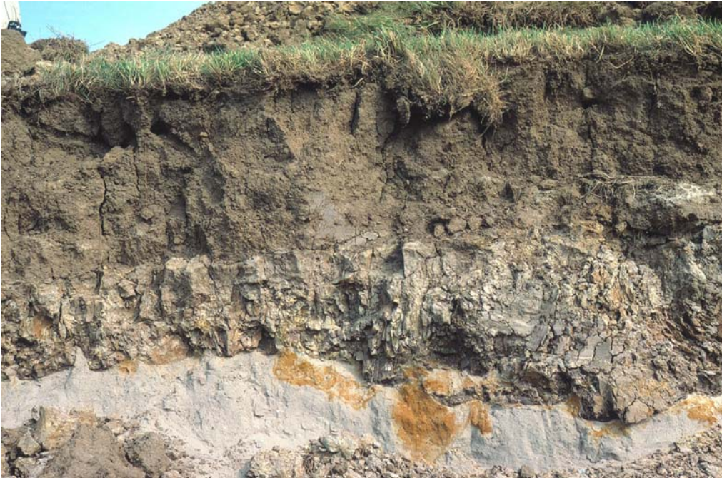
Figure 2.3B: Soil structure of clay in dikes. The photograph shows the influence of burrowing animals and root penetration up to 0.7 m deep. The structure underneath is the result of changes in moisture content.
