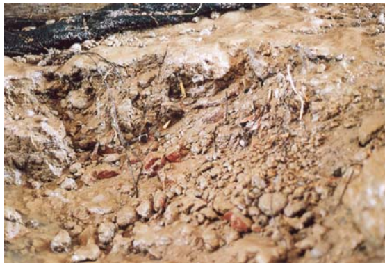
Figure 3.7: Damage caused by erosion of lumps from a clay layer with soil structure formed under a stone setting. The clay is in the form of lumps eroded out of a hole that is 0.4 m deep. Some lumps show brown patches due to iron compounds.
