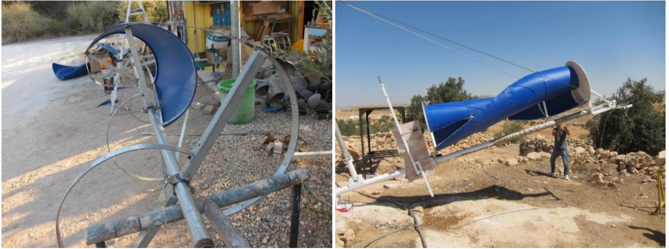
Figure 16 (left): Production of the Savonius Helical rotor using barrels and a metal frame. Figure 17 (right): Installation of the Savonius helical rotor
