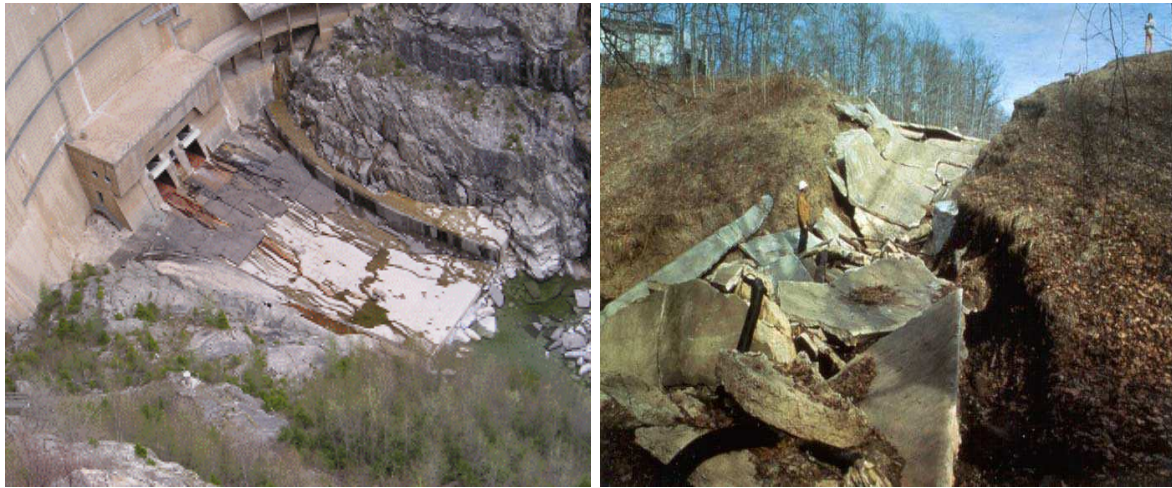
Figure 1-6. Plunge pool at Gebidem dam (left) [1]. A spillway failure caused by erosion, Harrington, 2012 (right).
