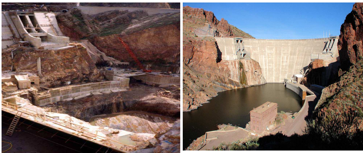
Figure 1-8. Spillway and plunge pool Theodore Roosevelt dam in during and after construction, Phoenix, Arizona, United State, 1996, [4].
