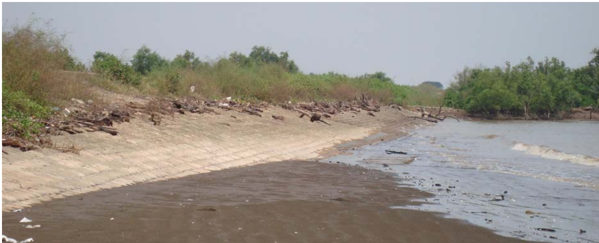
Figure 2: Example of a dike revetment recently constructed in Vietnam because of a disappearing mangrove forest
