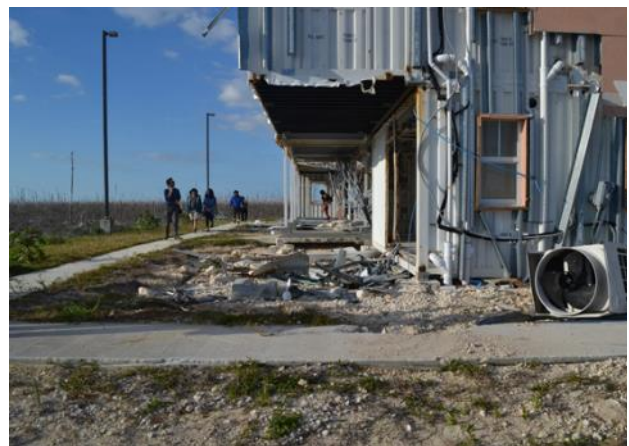
Fig 35: Destroyed dorm of the university campus.
