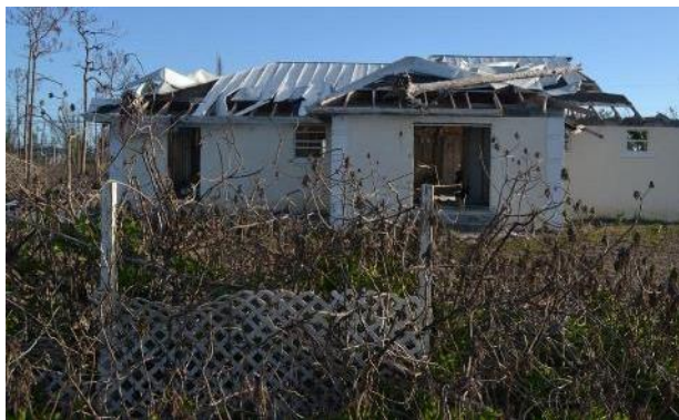
Fig 38: The outside of a house destroyed by Hurricane Dorian, damaged by water and wind picture taken 4 months after Dorian.
