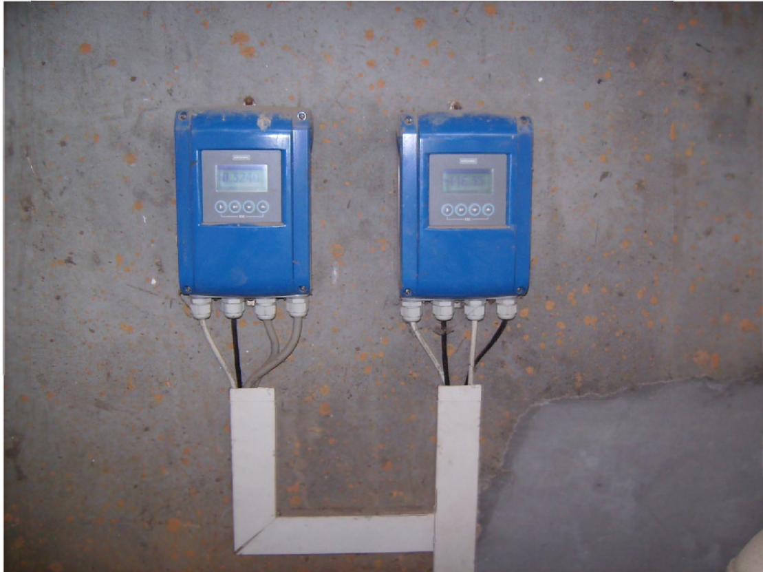
Figure 8 Flume Discharge Meter (Electromagnetic Flow Meter)
