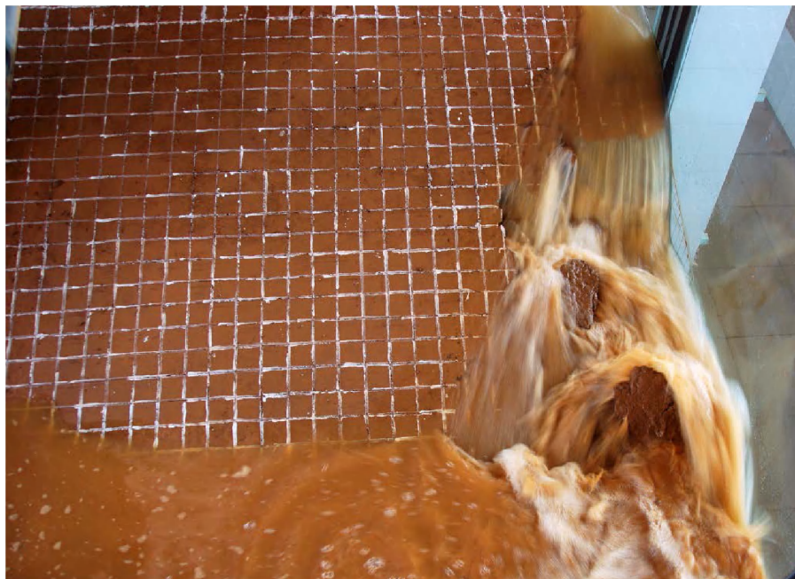
Figure 39 Photo of Headcut Erosion
