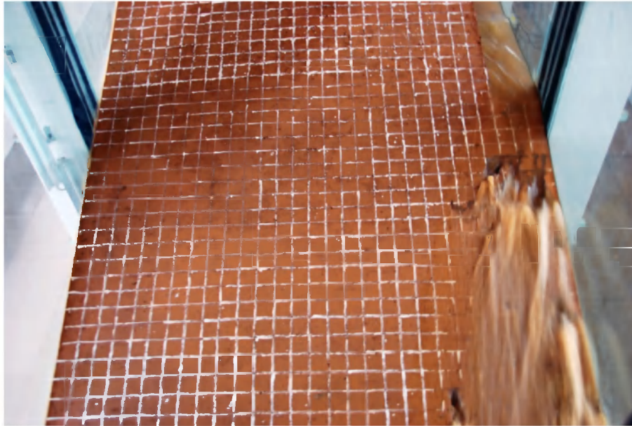
Figure 38 Surface Erosion at the initial phrase of breach
