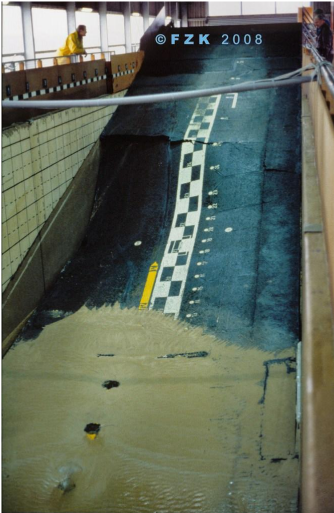
figuur 3.1 Ingestorte asfaltbekleding in GWK, Hannover
