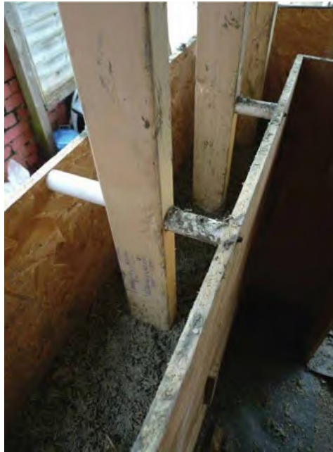
Fig.4: A softwood frame buried centrally in the wall is the standard design.
