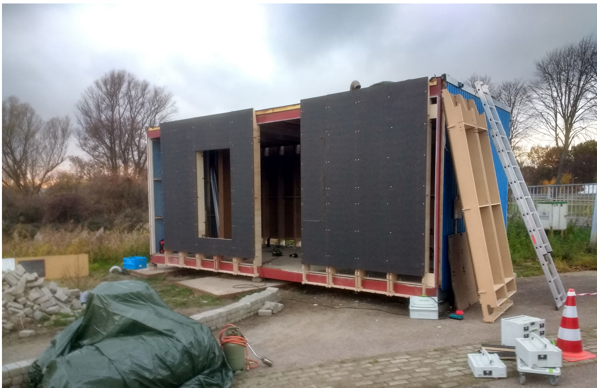
Figure 114: Outside photo during the construction of the tiny house with several wall components installed on the red frame.
