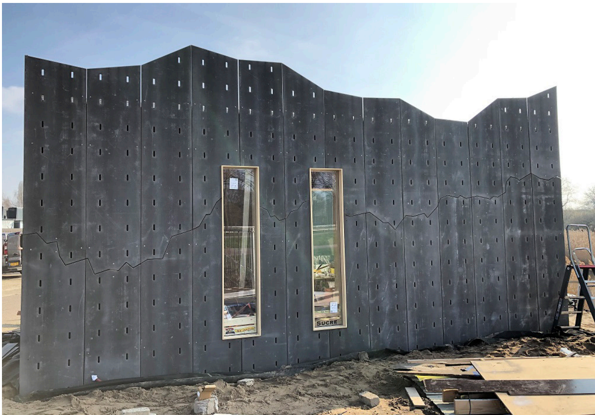
Figure 116: Photo of the exterior of the tiny house when construction is almost finished. Adapted from: Mertens (2019).
