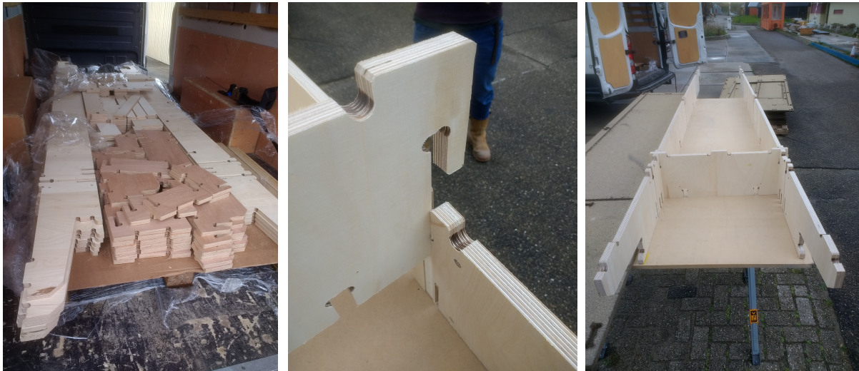
Figure 113: Three photos made during the on-site assembly day. From left to right: a stack of elements, a horizontal beam sliding into a vertical beam and an overview of the partially assembled wooden frame.
