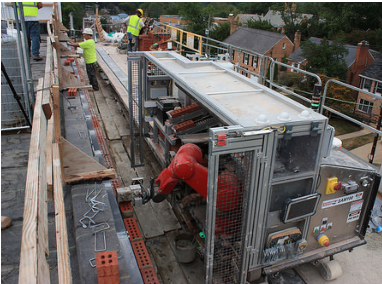
Figure 13: The robot SAM-100 is laying bricks on-site to construct the façade of The Lab School of Washington, DC. Reprinted from: Construction Robotics (n.d.).
