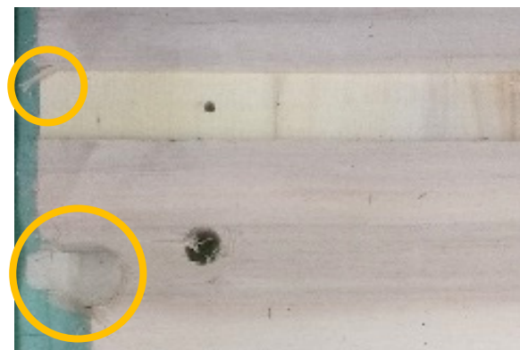
Figure 150: Photo of the bottom part of the right vertical beam of section one. The small circle highlights a splinter sticking out. The big circle marks a very thin layer of wood that should have been milled out.
