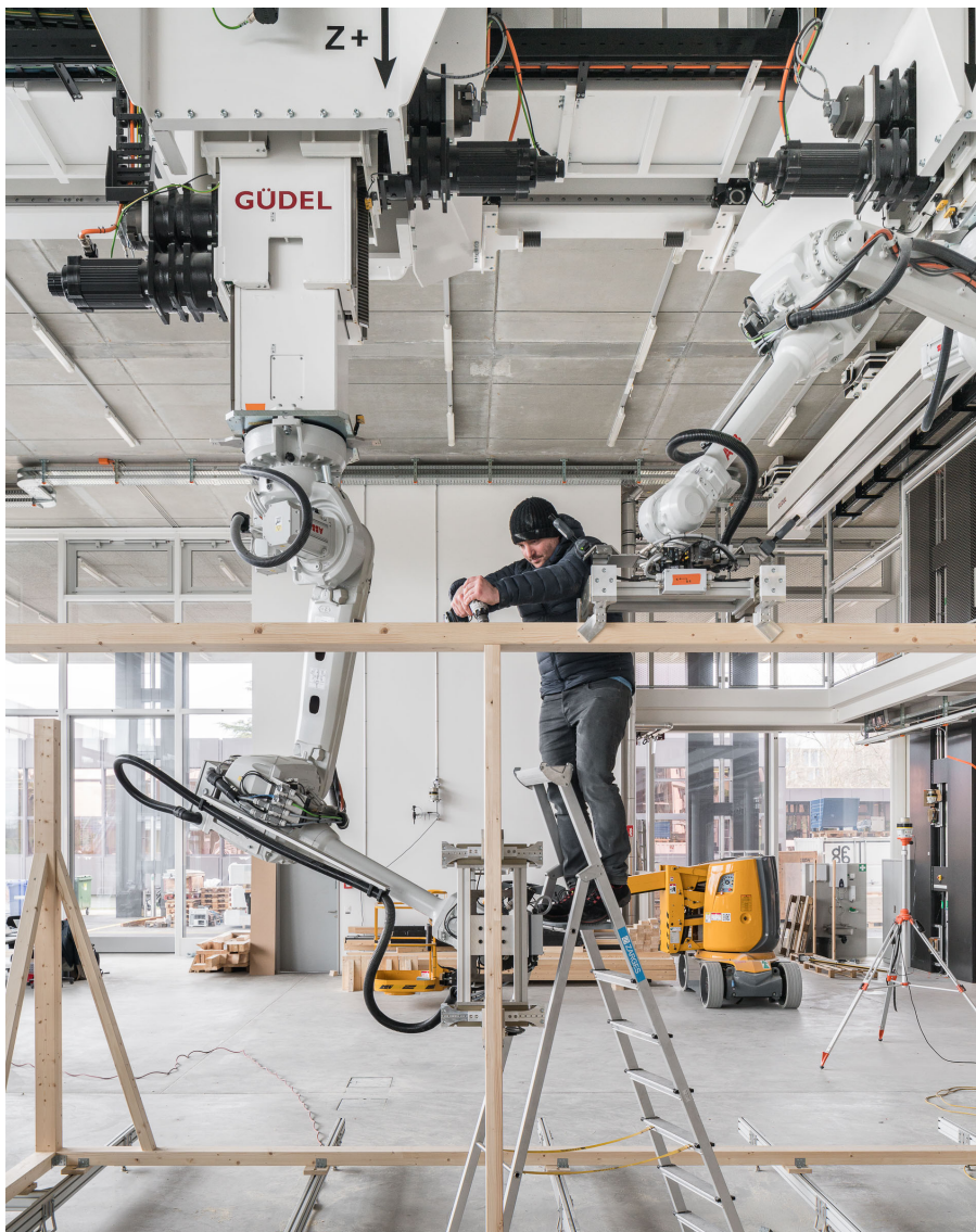
Figure 21: Worker fastens beams together while robot arms hold them in place. Reprinted from: ETH (2019).
