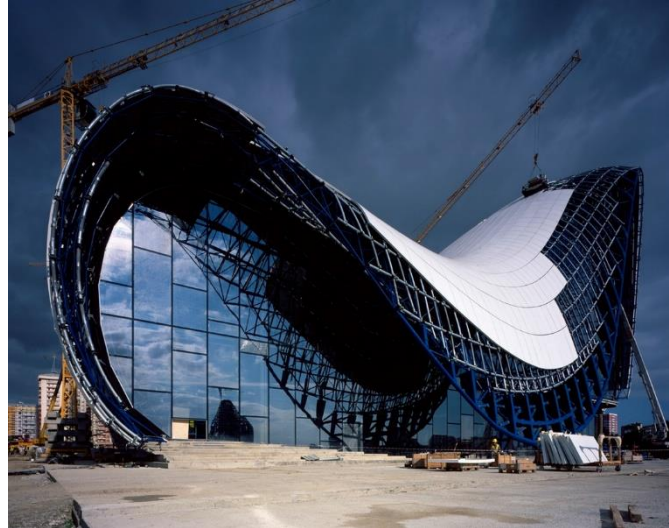
Prefab double curved panels are fitted to the underlying structure at the Heydar Aliyev Cultural Centre ( http://www.gizmag.com/zaha-hadid-heydar-aliyev-center-baku-azerbaijan/32783/ )
