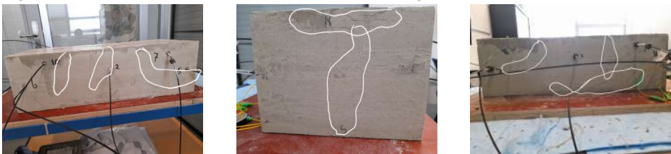
Figure 6.2: Cracks developed on concrete after curing
