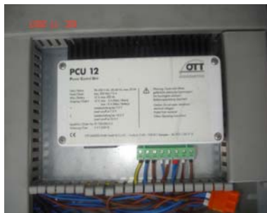
Power Control Unit - PCU
