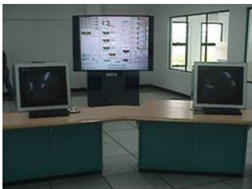
Figure 4.15 Operator & Overhead Projection Workstations
