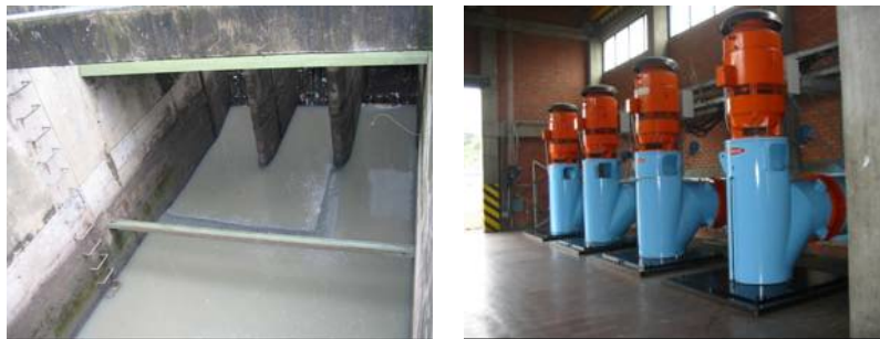
Figure 3.16 Floralia pumping station
