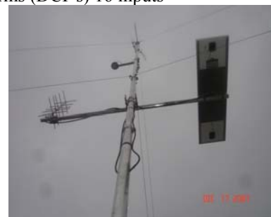
Solar Cell and Yagi Antenna
