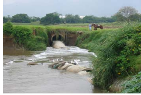
Figure 3.13 Margen Izquierda Collector discharge point, after collapsing in 2003.
