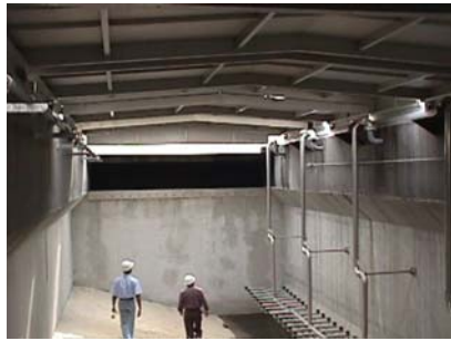
Figure 3.27 Aerated grit removal
