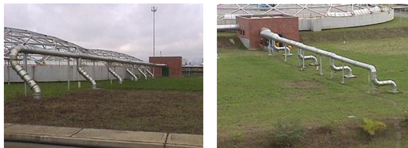
Figure 3.36 Odor control system - soil beds.
