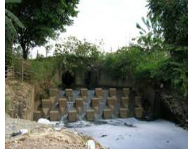
Figure 3.18 Discharge point Puerto Mallarino Pumping station
