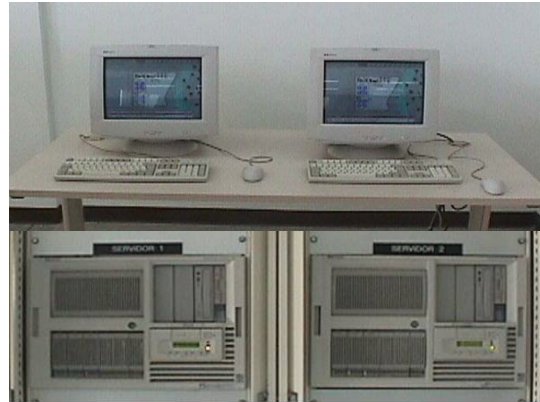
Figure 4.14 Mainframe and Back-up Servers
