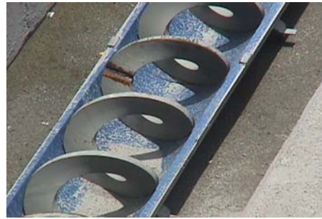
Figure 3.28 Sand removal system
