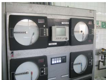
Panel of data recording for the purification water process at Puerto Mallarino
