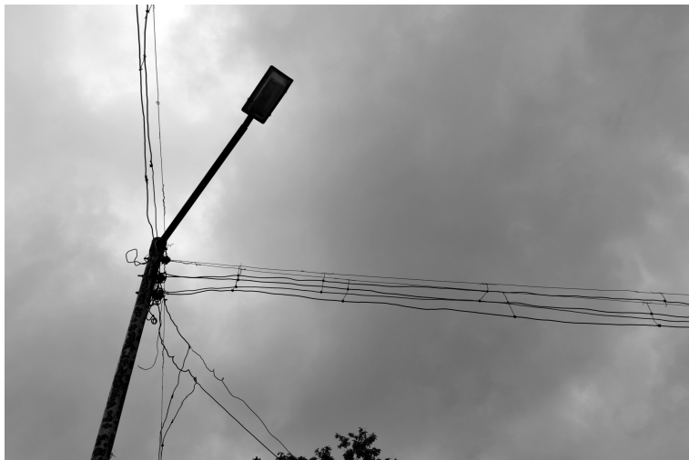
Figure 3.4 Power Distribution Network (PDN) with extra cables connected by the villagers.
