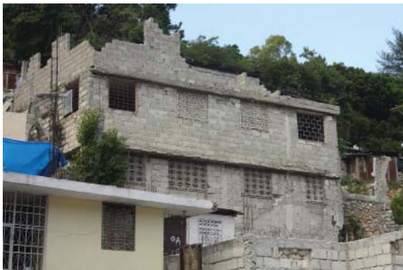
Fig. 5.19: Promotion of ventilation in the cement block houses, Villa Rosa, Port-au-Prince Source: Author
