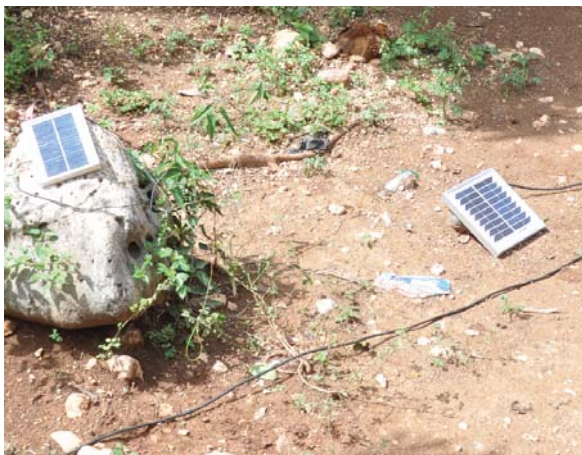
Fig. 8.9: PV cells to generate electricity in Villa Rosa (top) and Septieme Gerard (bottom). Source: Author
