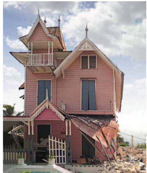
Fig. 5.22:Gingerbread house next to a collapsed concrete house Source: Langenbach, 2010, pp. 40
