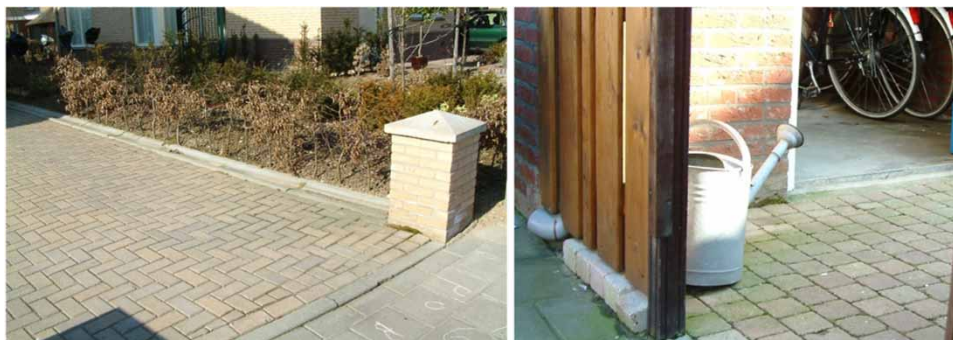
Figure 1 | Two cases (#13 and #15) of technical failures in SUDS with a failing function of conveyance. Left: an obstacle interferes with the transport of water by an open gutter. Right: due to insufficient slope of the garden, the storm water flows into the shed.
