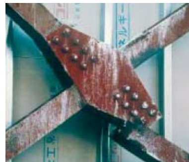
Figure 3.27: Truss bracing failure [Bachmann, H., 2003]
