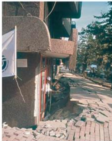
Figure 3.30: Soil liquefaction [Bachmann, H., 2003]
