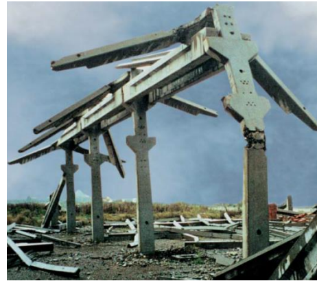
Figure 3.28: Connection failure prefabricated building [Bachmann, H., 2003]
